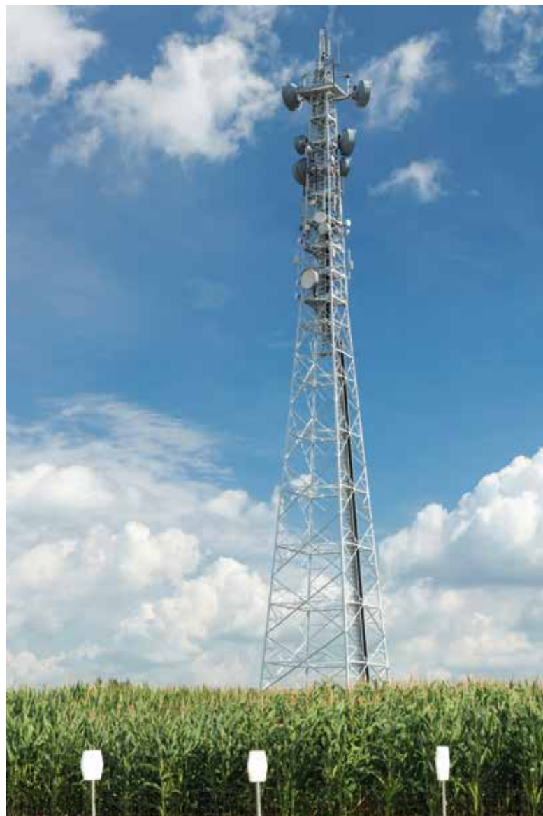
BELOW: Communications tower.
